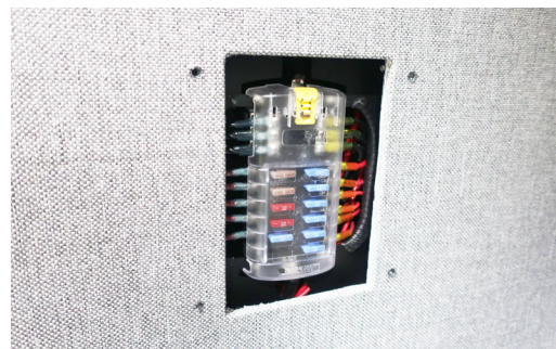
House 12-Volt Fuses (Located on right side twin bed cabinet at rear) -Typical View
